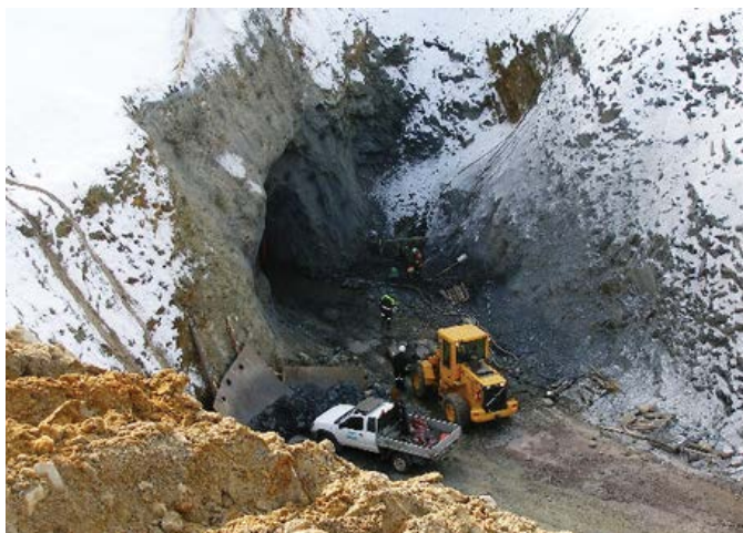
Picture 7.1: Testing prior to the possible reopening of the Hannukainen mine, Finland.
